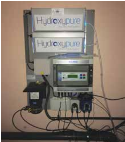
Hydroxypure cleverly responds to different demands such as hot weather, high bather loads, rain and water top-ups; in fact the Hydroxypure system automatically adjusts dosing requirements to suit.
